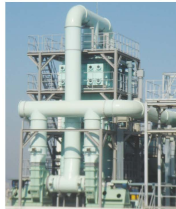
Large-sized WET-EP System (Roof Outside the FAB)
